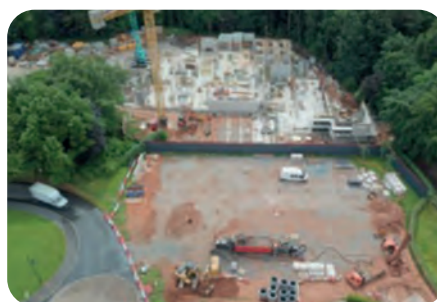
Figure 5 - Riddell Hall geothermal project
