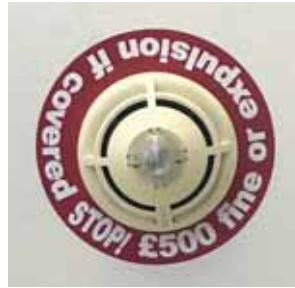
Smoke/heat detector in room
