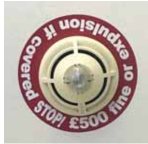
Smoke/heat detector in room
