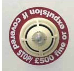
Fig. 2 smoke/heat detector in room
