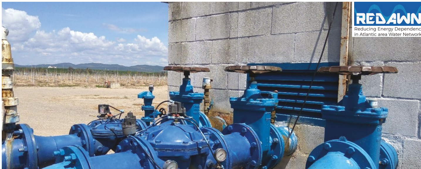
Site of demonstration micro-hydro power plant in the irrigation sector, Genil River irrigation district, located in the Guadalquivir river basin, Andalucia, Spain.
