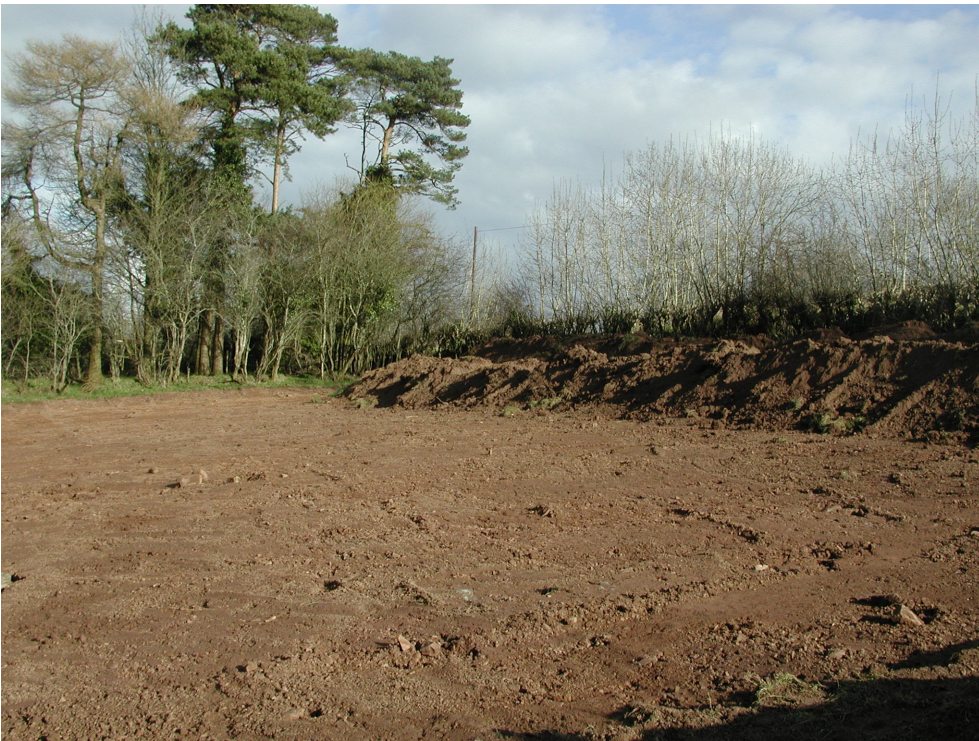
Plate 2: View of southern part of site, in vicinity of Point B, after excavation to subsoil level (C203).
