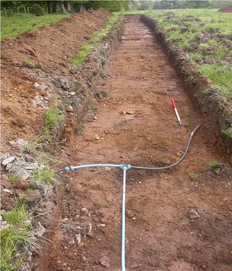
Plate 1: View of Trench A from west, after excavation to surface of subsoil (C104).
