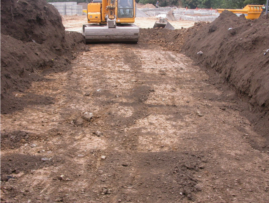
Plate 9: View of topsoil stripped area in south of site after removal of spoil heap. Note, some relict traces of topsoil remain along the line of the bucket.
