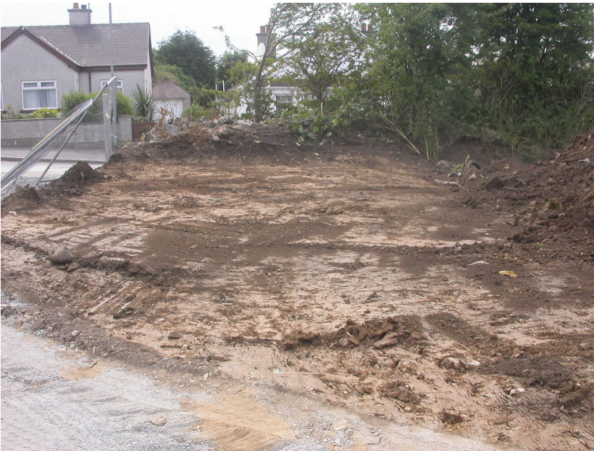
Plate 8: View of topsoil stripped area in south-west of site after removal of spoil heap.
