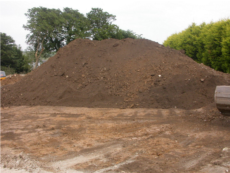
Plate 10: View of topsoil stripped area in south of site. Note, some relict traces of topsoil remain.
