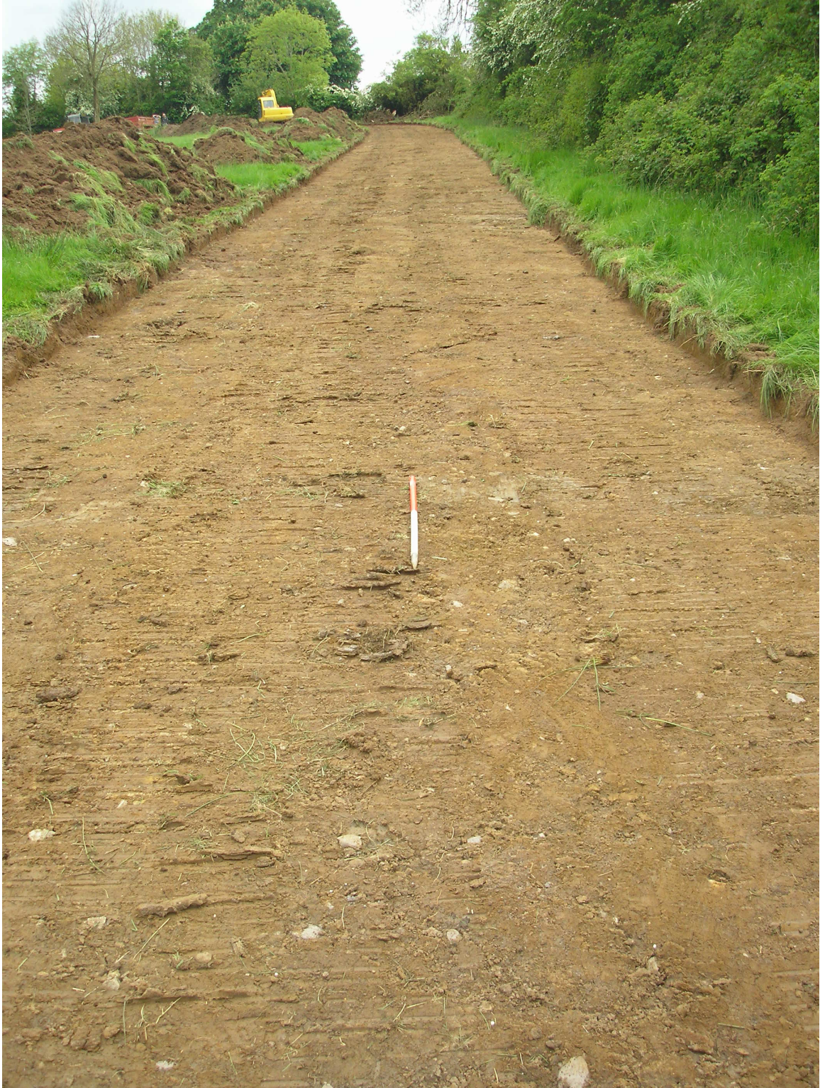
Plate One: Access lane following excavation to the surface of the natural subsoil (Context No. 103), looking south-west.
