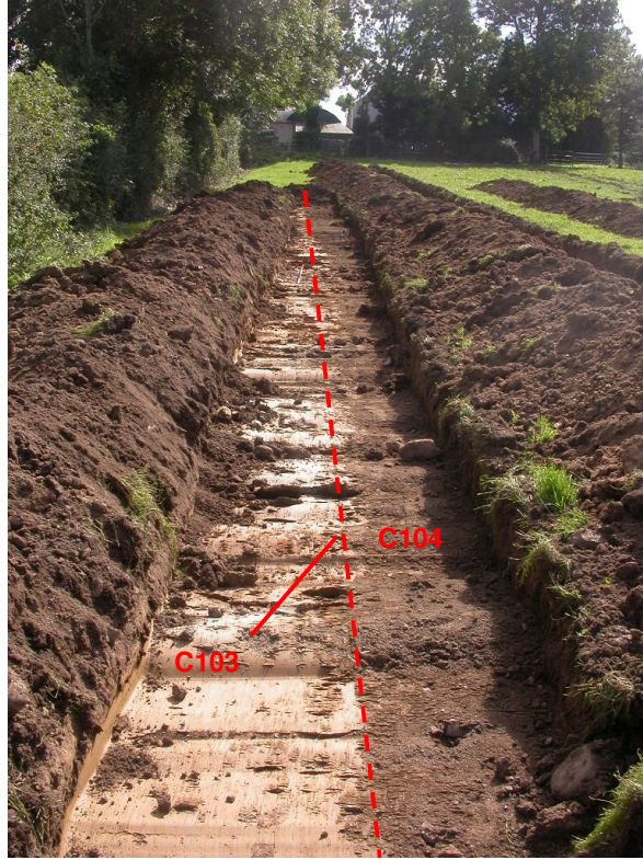
Plate Three: Trench One following excavation to subsoil (Context No. 108), looking south-east
