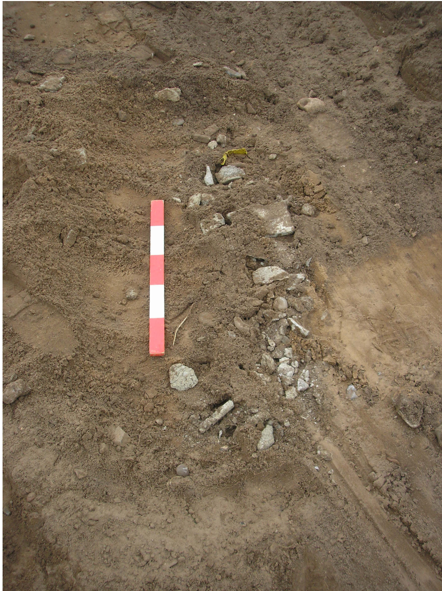
Plate 3: Detail of stone fill (Context No.104) of the cut (Context No. 103) for the electric cable.
