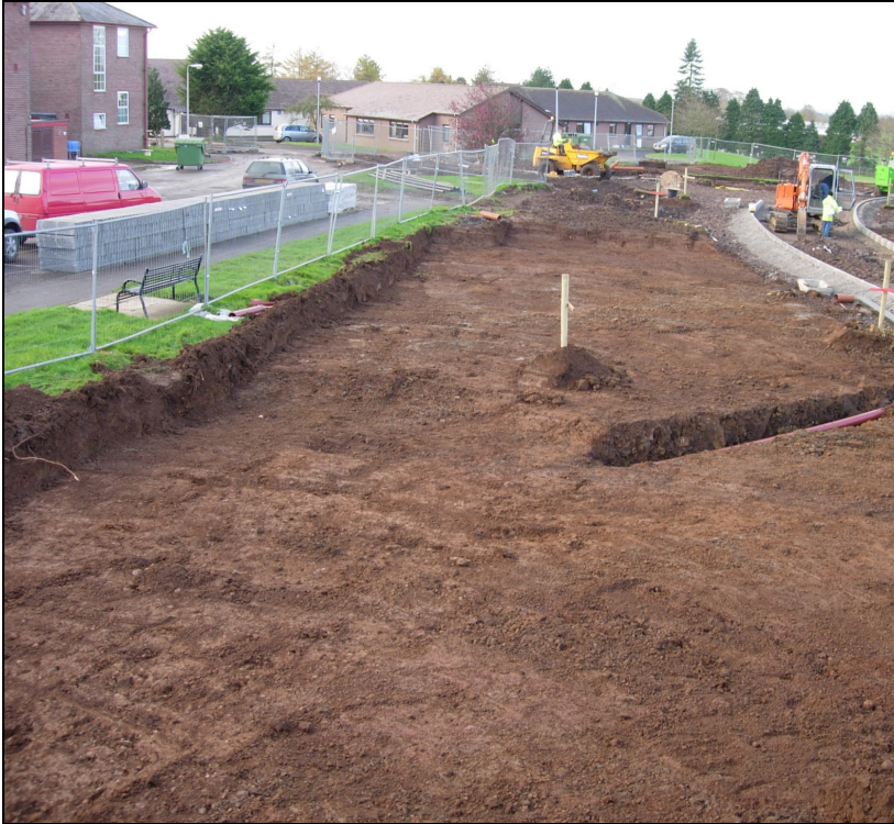
Plate 7. The excavated area at completion of the monitoring work. (The apparent arcs in the foreground are due to the tracks of the mechanical excavator) (Facing south-east).
