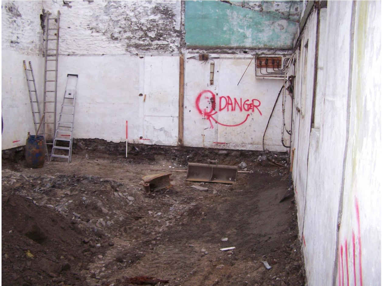
Photo 1: West end of building after removal of floor and reduction of ground level.
