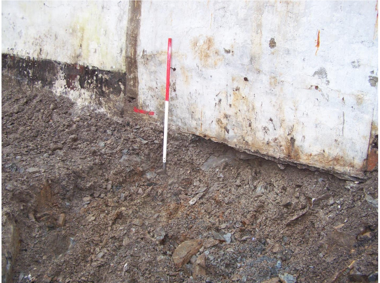
Photo 3: View of the interface between the battered wall (left of photo) and the plain wall (right of photo). Note the difference in the foundation materials of the two sections of wall.
