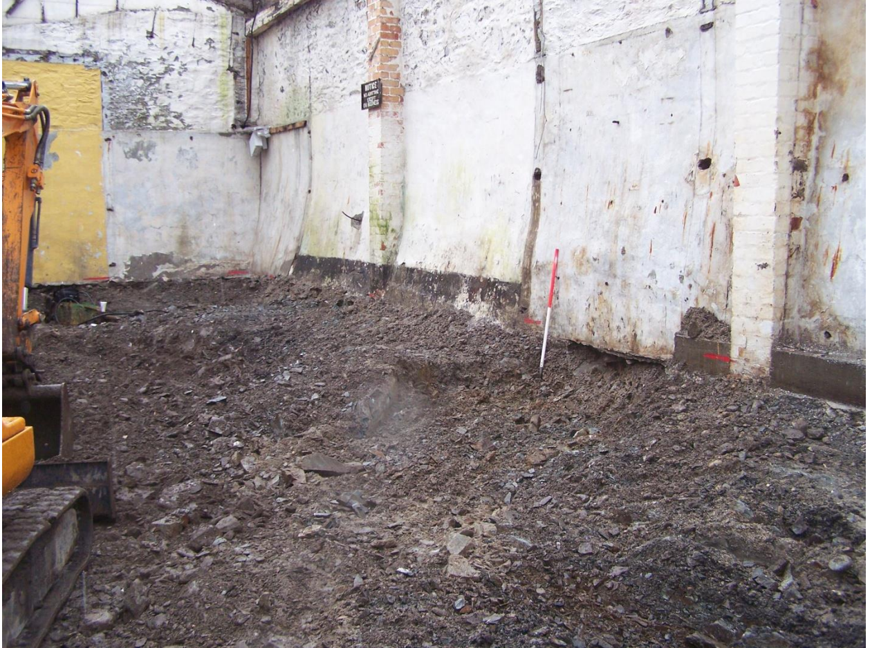
Photo 2: View of east end of building after removal of floor showing bedrock. Note change in wall type from battered wall sitting on bedrock, at east end, to plain wall founded on rubble infill at west
