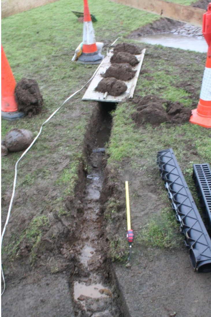
Plate 8 The narrow trench linking the excavation trench and tarmac path to host the artificial drainage pipe.
