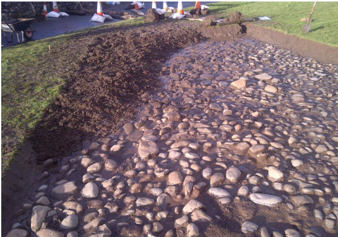
Plate 11 The northern end of the excavation trench with the north-western corner (where the cobbles had been previously removed) back-filled.
