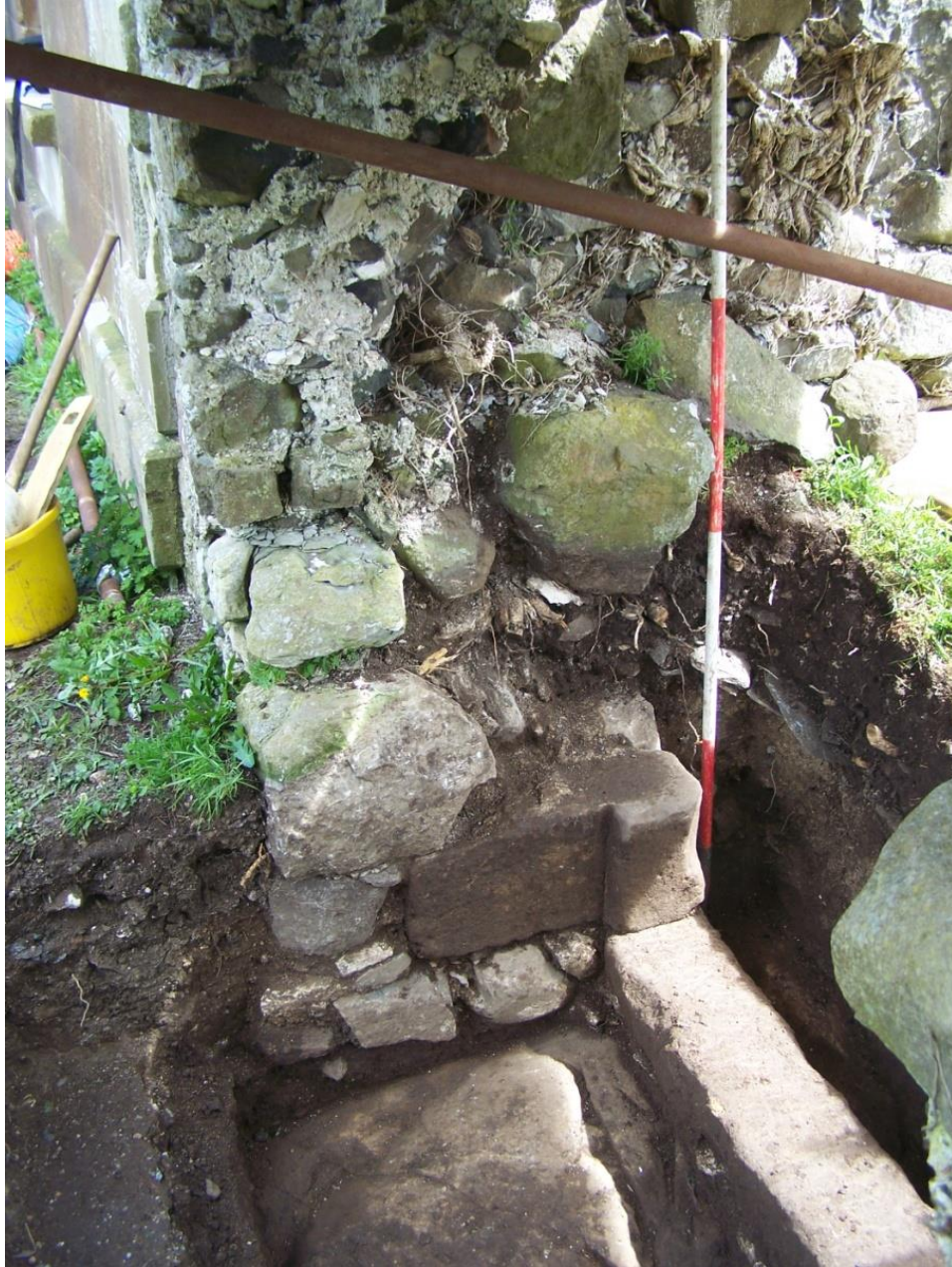
Plate 4: Photo of the in situ door-jamb (Context No. 110) and threshold (Context No. 108) post excavation, looking south-east.
