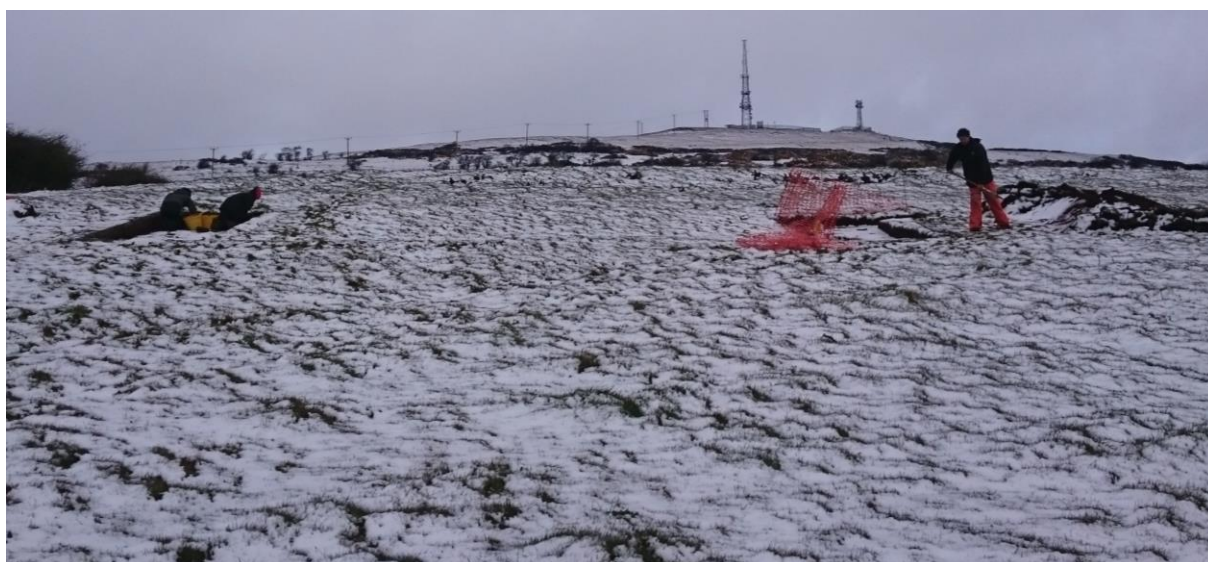
Plate 7. Squire's Hill, Belfast, 28th April 2016. Backfilling the trenches, with Trench 1 to the left of the photo and Trench 2 to the right. Photo taken from south.
