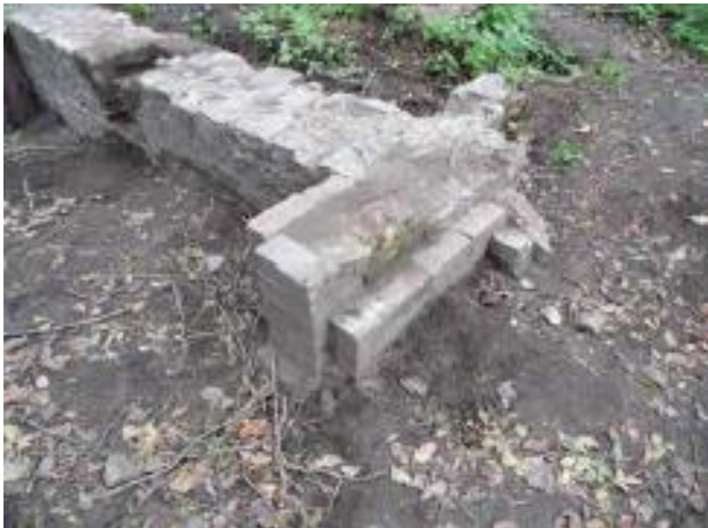
Pl 5: Detail of north opening west side taken from southeast showing brick pier addition at wall W1 (M. Conway, NT)
