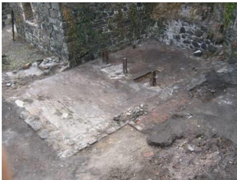
Post-excitation view of the retort area of a domestic gasworks. National Trust
